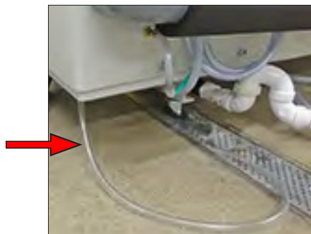
Figure 6.7i: Bubble tower drain connection.
