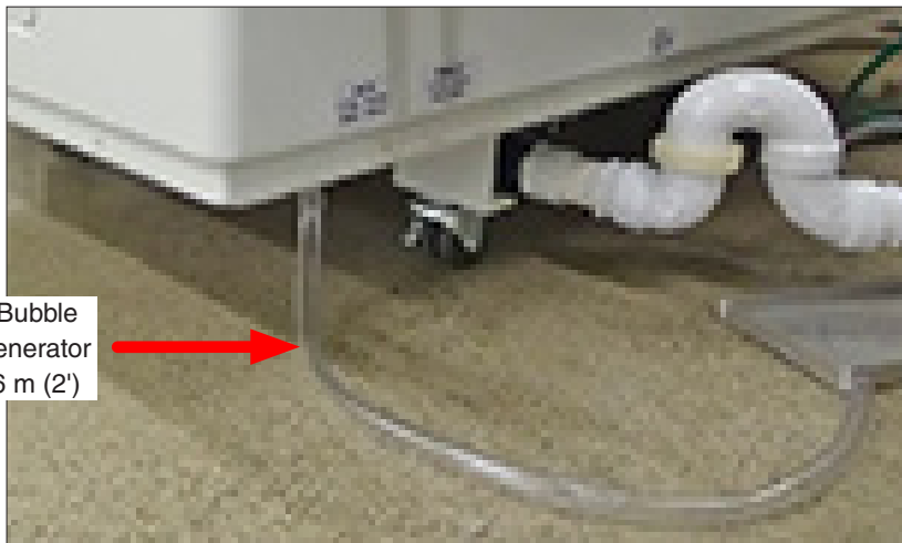
Figure 5.8f: Bubble tower/vapor generator drain connection.
